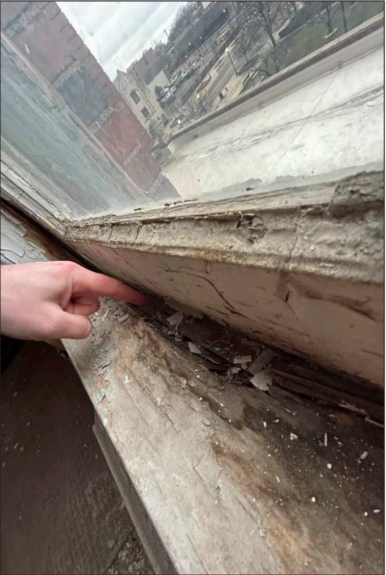
62. W25 – West Elevation, Fifth Floor, detail of deterioration at jamb and bottom sash. Note separation of jamb to interior casing.
