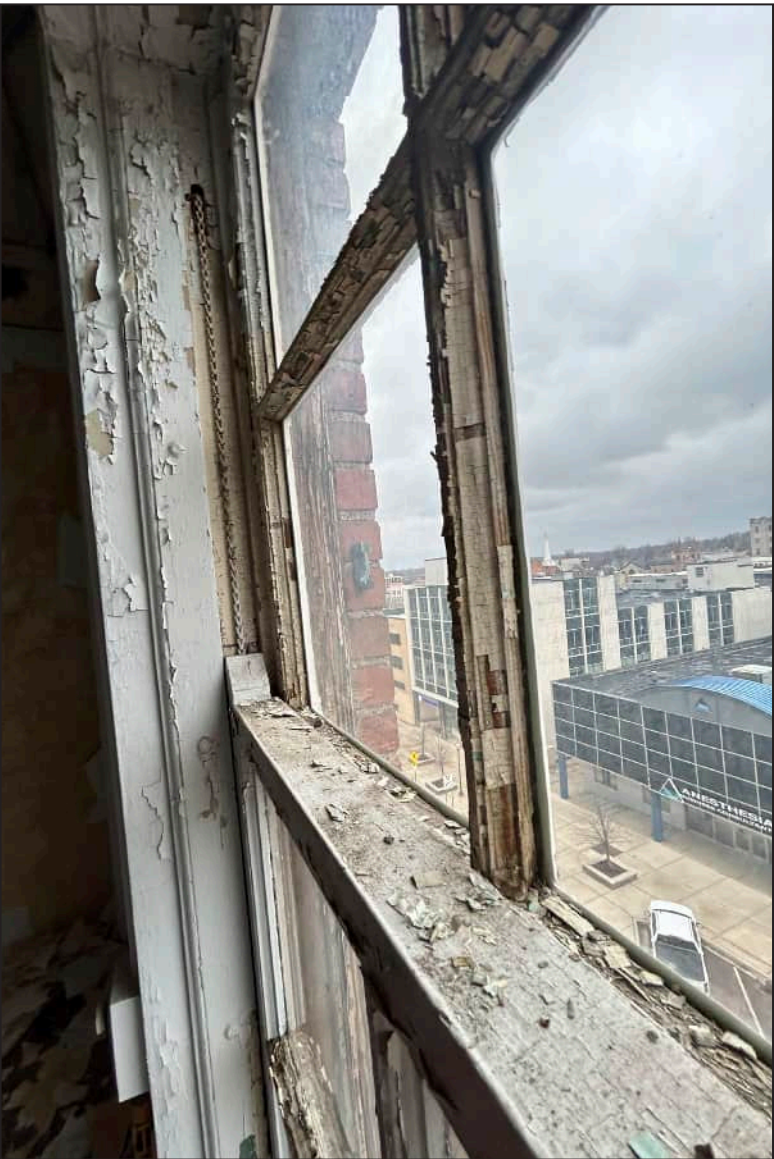
27. S27 – South Elevation, Sixth Floor, detail of deterioration of mullions, meeting rail, and jamb.
