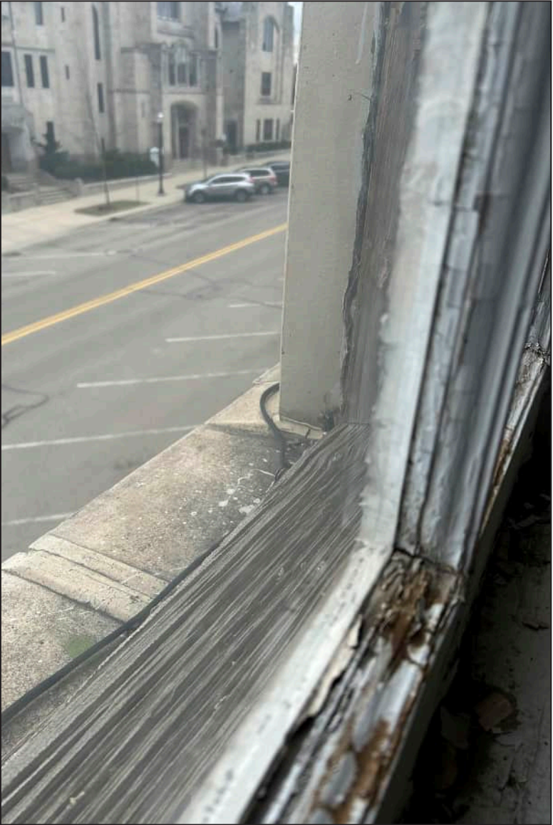
6. S06 – South Elevation, Third Floor, detail of rotting at bottom sash. Note deterioration of wood at exterior framework.
