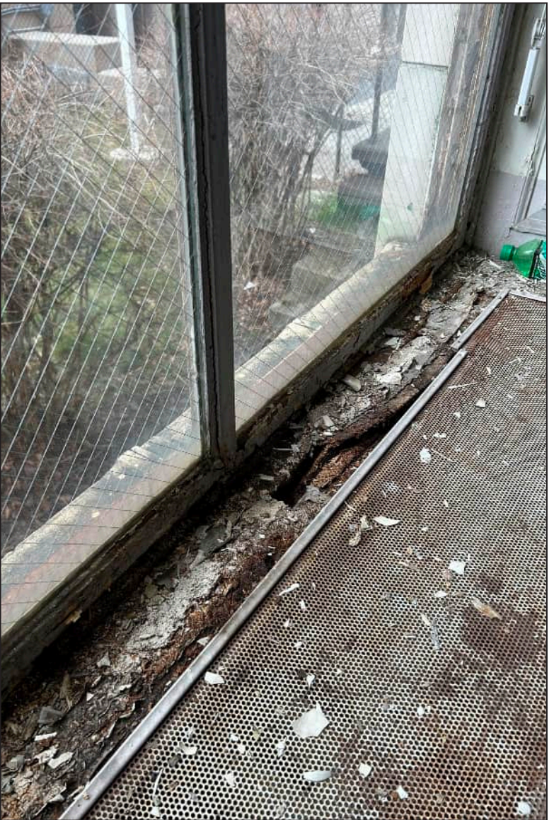
45. W08 – West Elevation, Second Floor, detail of deterioration at bottom sash. Note separation of bottom sash with sill.
