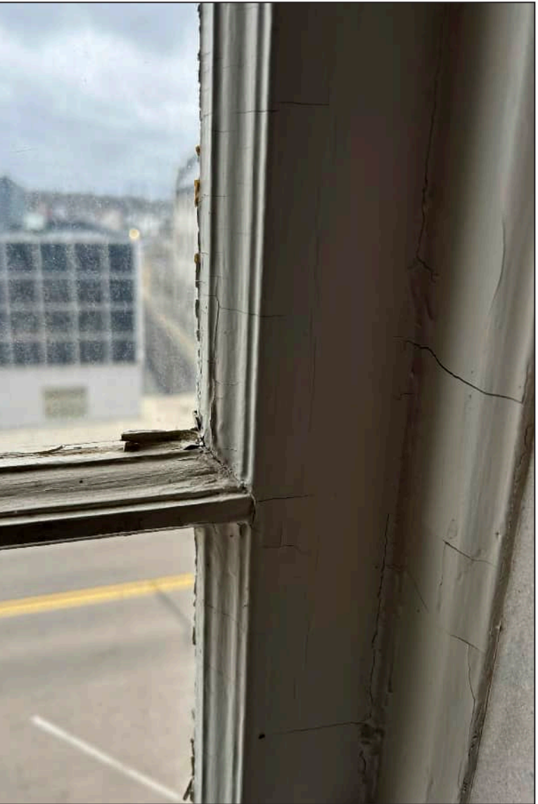
20. S20 – South Elevation, Fourth Floor, detail of rotting at mullion.
