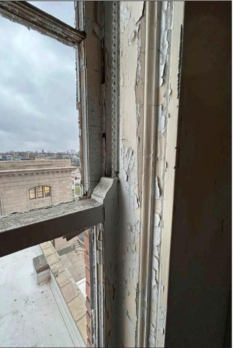
60. W23 – West Elevation, Fifth Floor, detail of deterioration at jamb, meeting rail, and mullion.
