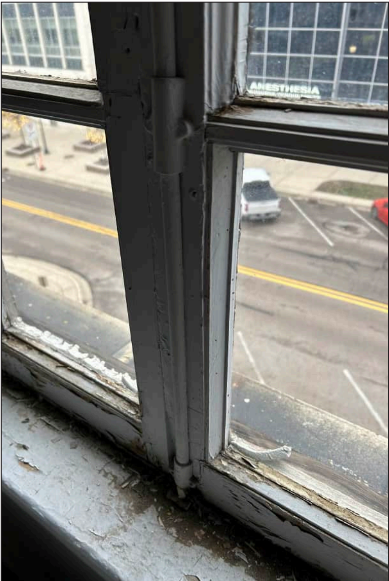
17. S17 – South Elevation, Fourth Floor, detail view of deteriorated mullions, rotting at bottom sash.
