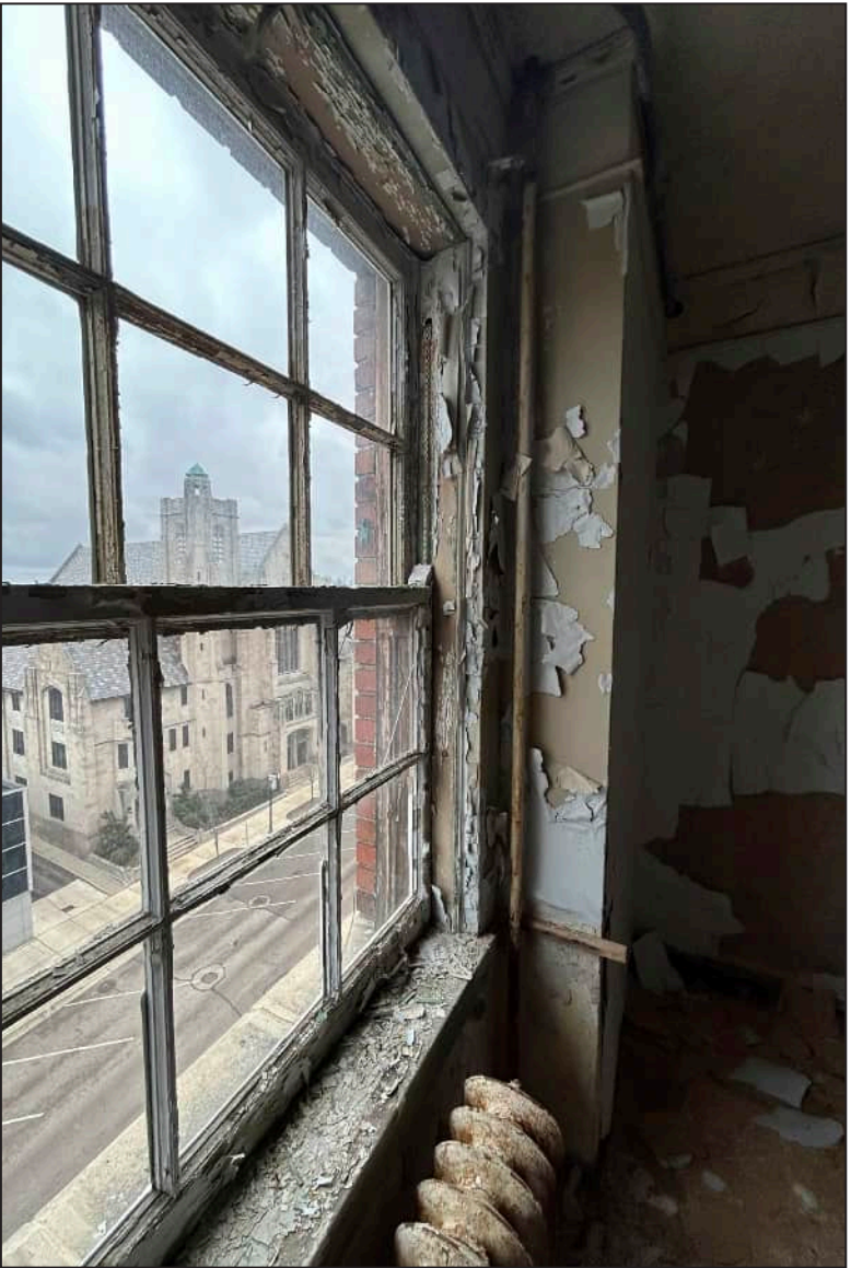
30. S30 – South Elevation, Sixth Floor, detail of deterioration of mullions, meeting rail, upper and bottom sashes, and jamb. Note deterioration at exterior framework.
