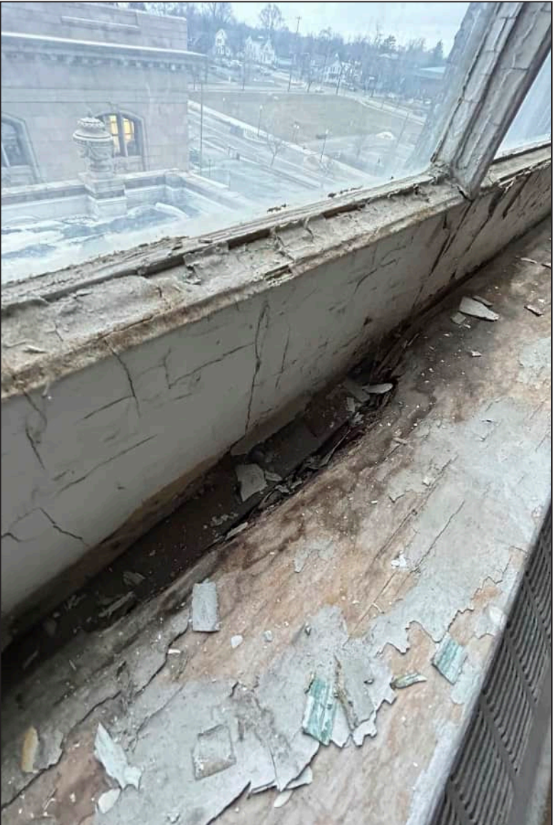
63. W26 – West Elevation, Fifth Floor, detail of deterioration at jamb and bottom sash. Note separation of jamb to interior casing.
