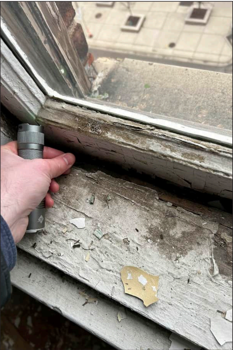
37. S37 – South Elevation, Eighth Floor, detail of rotting at jamb and bottom sash. Note separation of frame to tracks and exterior wood deterioration.
