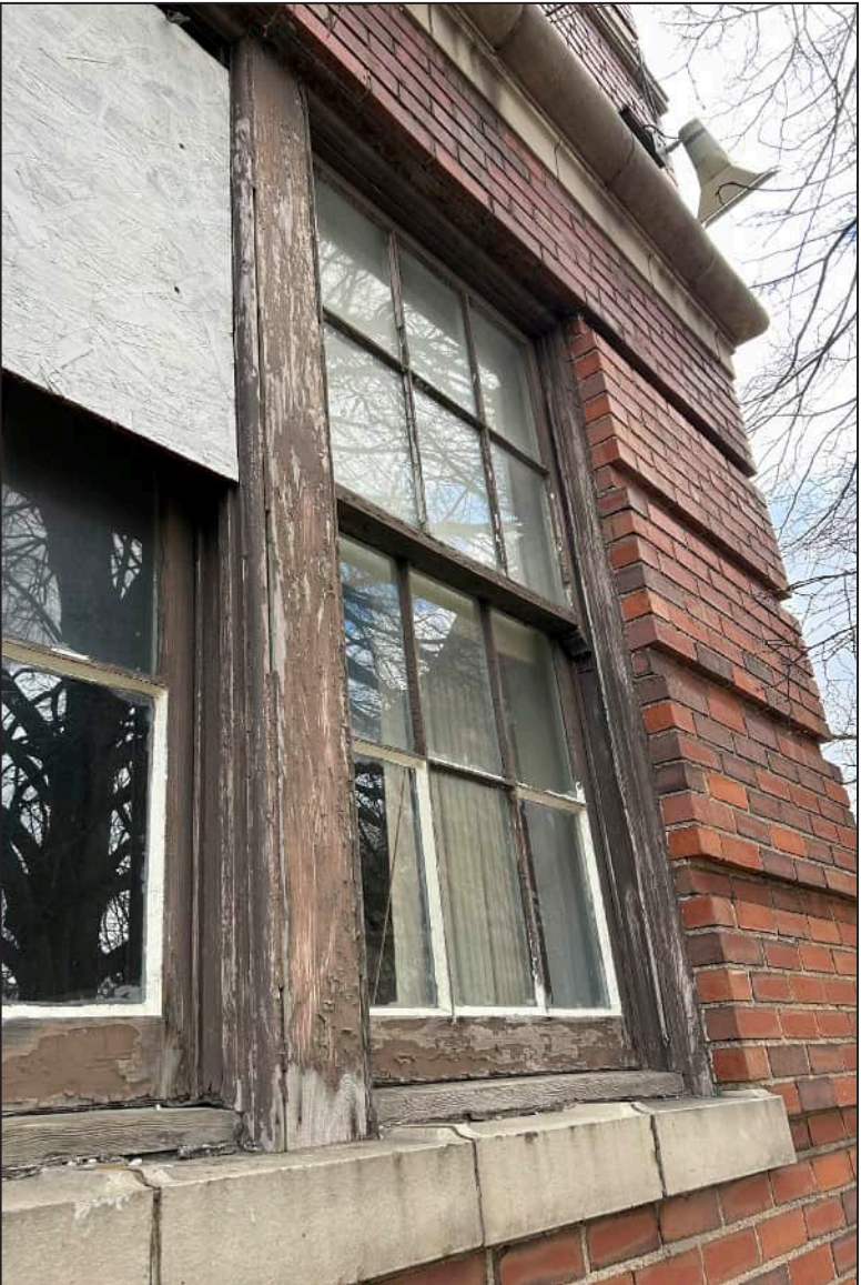
55. W18 – West Elevation, Second Floor, detail of deterioration and rotting at exterior framework and center muntin.
