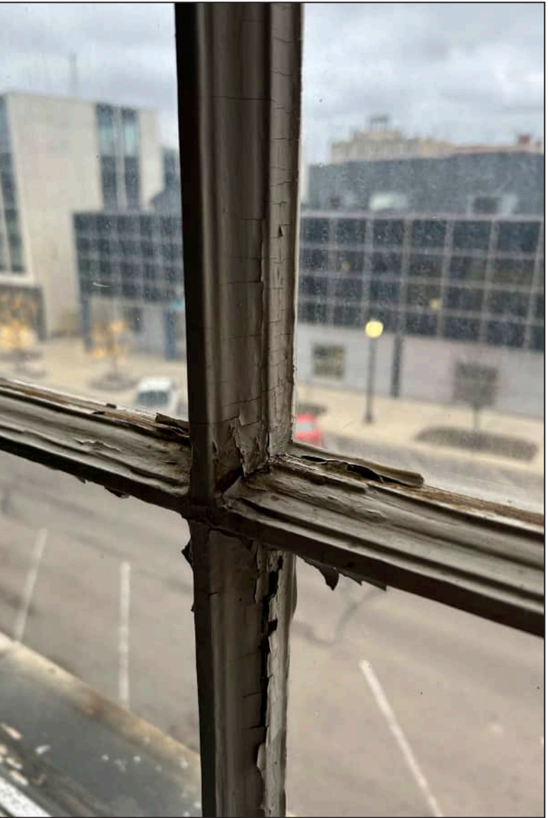
14. S14 – South Elevation, Fourth Floor, detail view of deteriorated mullions, general rotting throughout the framework.
