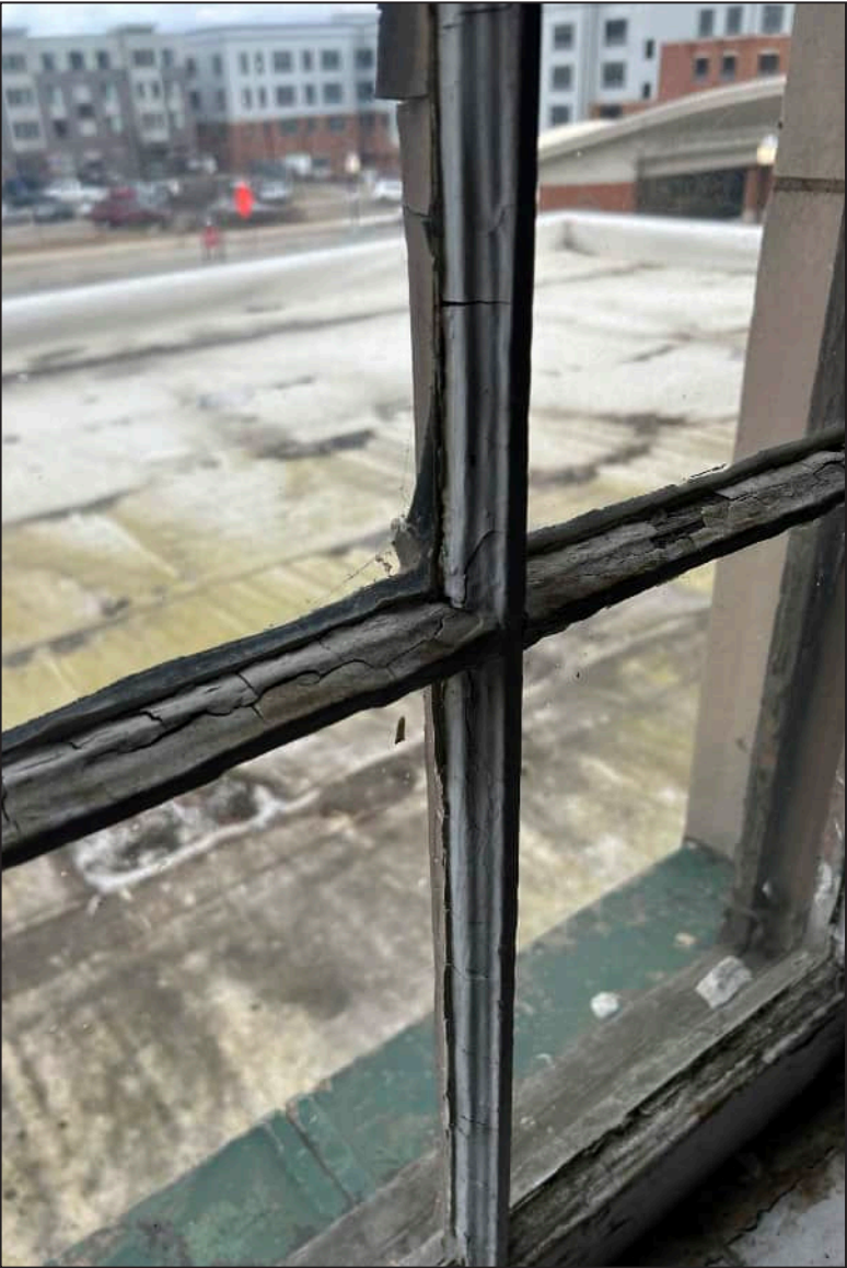
71. N05 – North Elevation, Fifth Floor, detail of deterioration of mullion.
