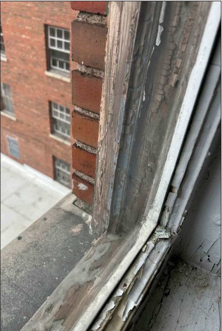
77. N11 – North Elevation, Eighth Floor, detail of deterioration of jamb and bottom sash. Note deterioration of exterior framework.
