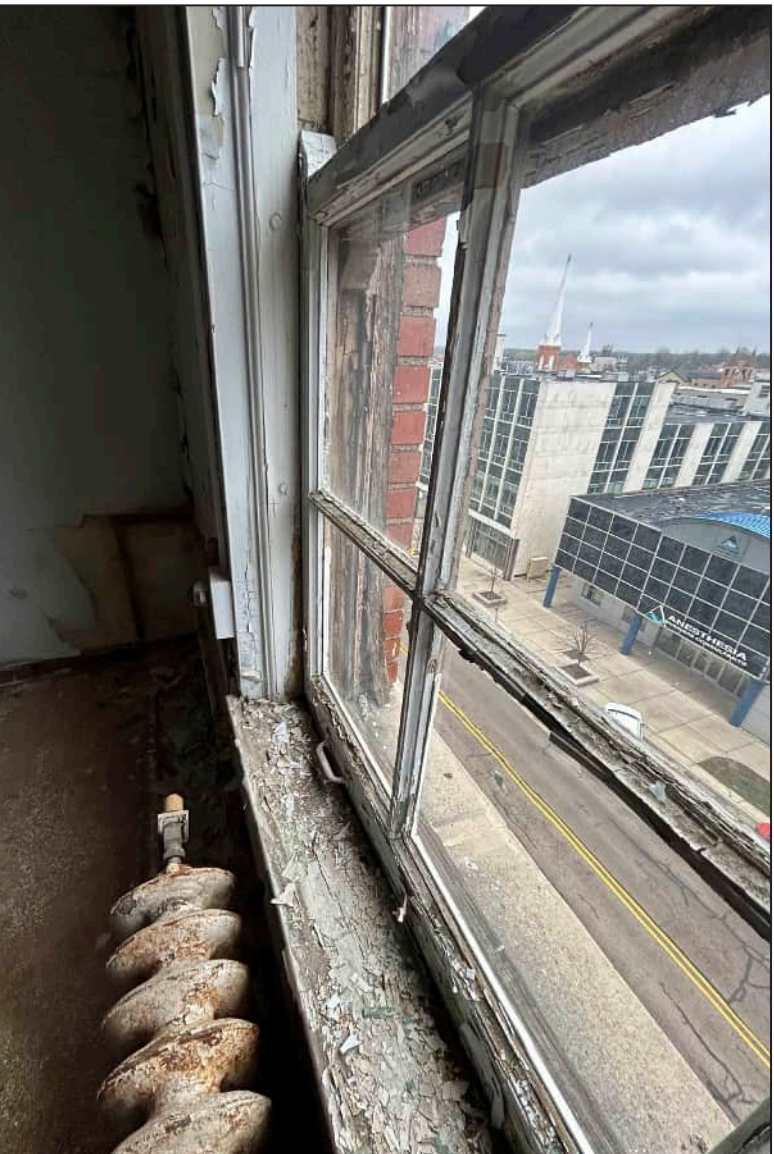
31. S31 – South Elevation, Sixth Floor, detail of deterioration of mullions, meeting rail, bottom sash, and jamb. Note deterioration at exterior framework.
