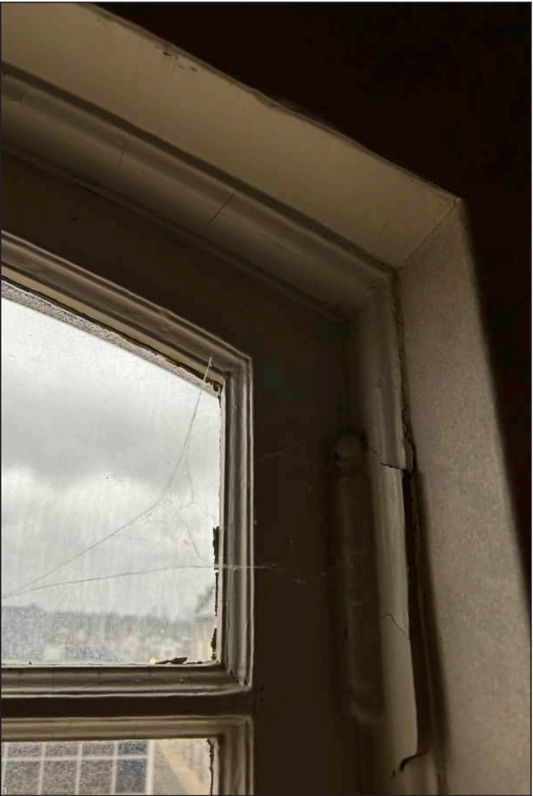
12. S12 – South Elevation, Fourth Floor, detail of altered interior trim at top of window.
