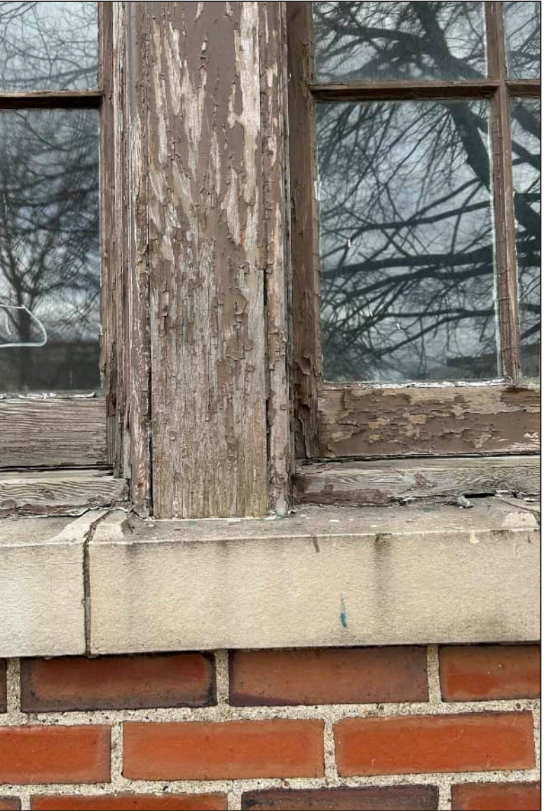
56. W19 – West Elevation, Second Floor, detail of deterioration and rotting at exterior framework and center muntin.
