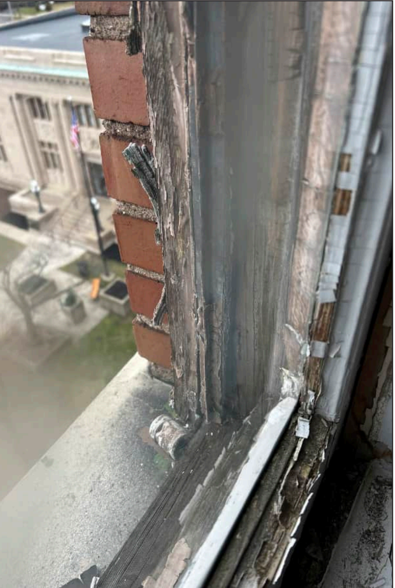
66. W29 – West Elevation, Eighth Floor, detail of deterioration of jamb and bottom sash. Note deterioration of exterior framework.
