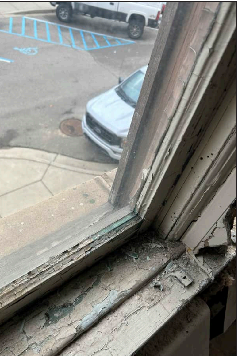
86. E09 – East Elevation, First Floor, detail of deterioration of jamb and bottom sash. Note deterioration of exterior framework.
