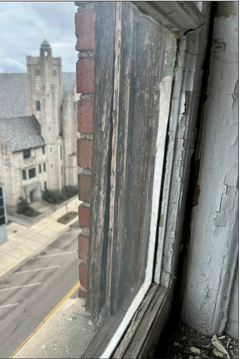
36. S36 – South Elevation, Eighth Floor, detail of deterioration of bottom sash and jamb. Note deterioration at exterior framework.
