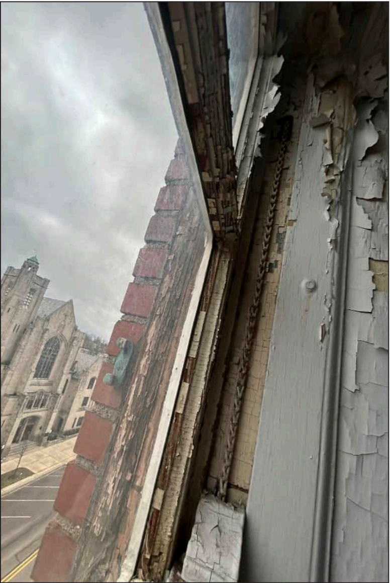
28. S28 – South Elevation, Sixth Floor, detail of deterioration of mullions, meeting rail, and jamb. Note deterioration at exterior framework.
