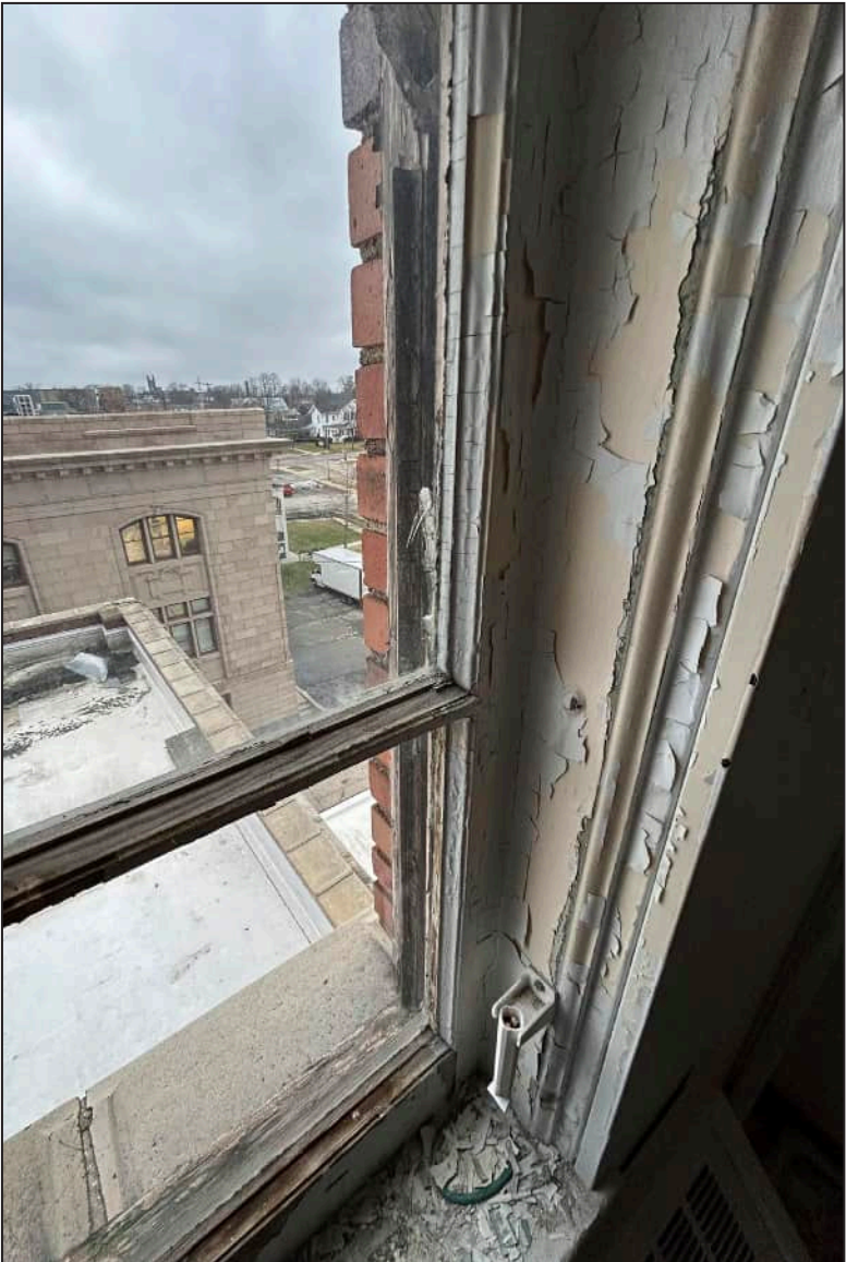
61. W24 – West Elevation, Fifth Floor, detail of deterioration at jamb, lower sash, and mullion.
