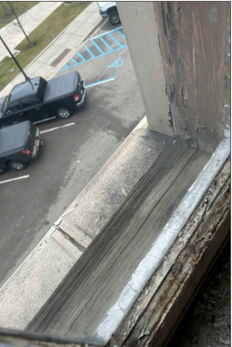
96. E19 – East Elevation, Fourth Floor, detail of deterioration of jamb and bottom sash. Note deterioration of exterior framework.
