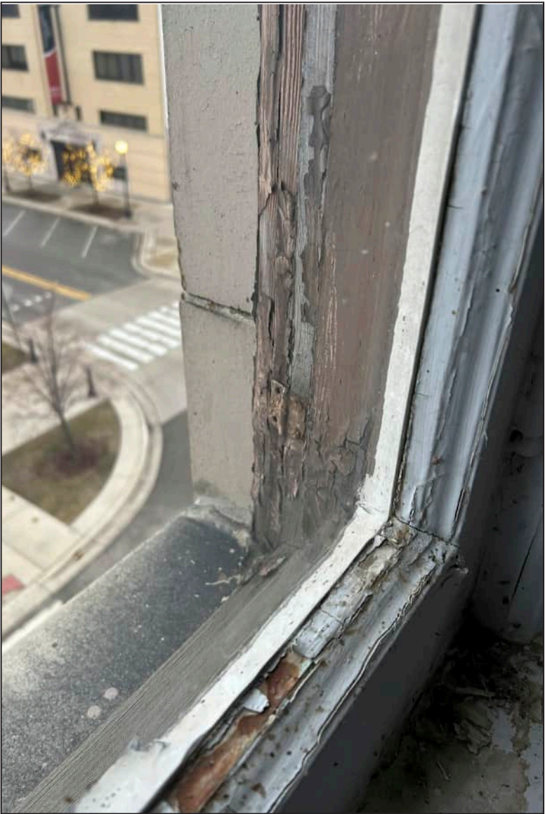
95. E18 – East Elevation, Fourth Floor, detail of deterioration of jamb and bottom sash. Note deterioration of exterior framework.
