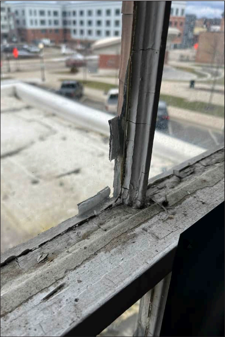
73. N07 – North Elevation, Fifth Floor, detail of deterioration of mullions and meeting rail.
