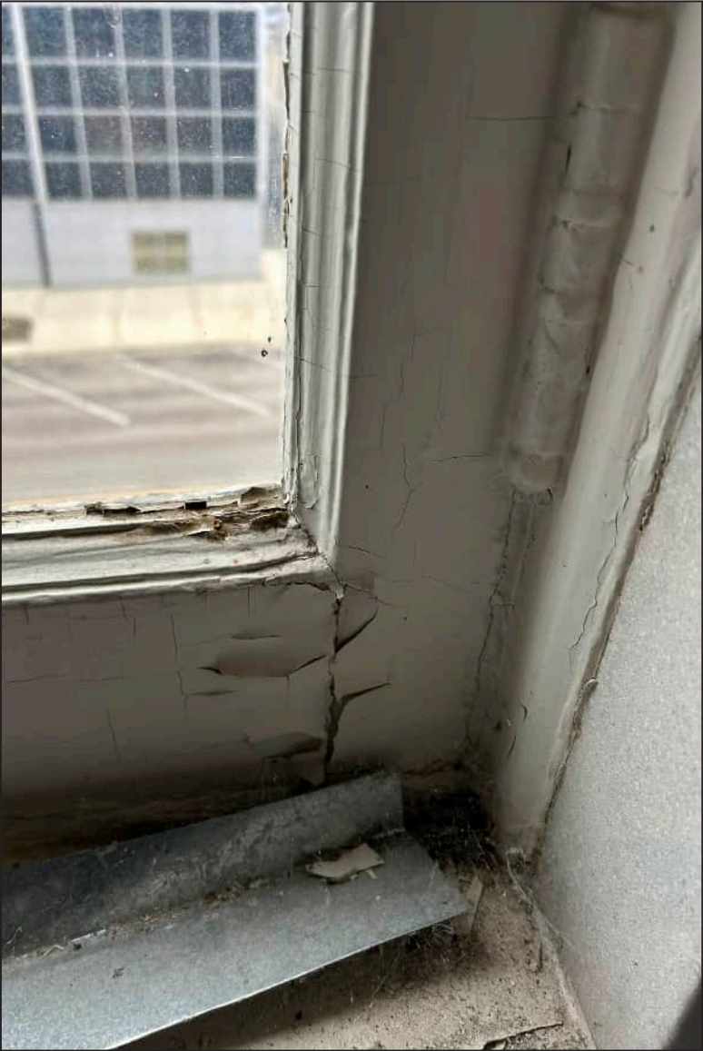
16. S16 – South Elevation, Fourth Floor, detail of rotting bottom sash, separation between jamb and bottom sash.
