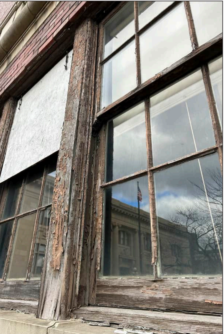
52. W15 – West Elevation, Second Floor, detail of deterioration and rotting at exterior framework and center muntin.
