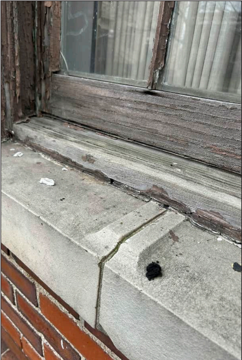
57. W20 – West Elevation, Second Floor, detail of deterioration and rotting at exterior framework.
