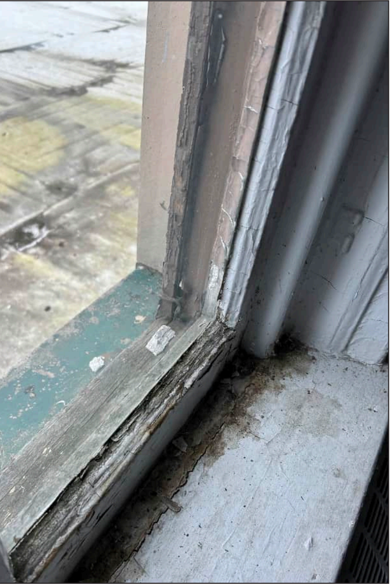
72. N06 – North Elevation, Fifth Floor, detail of deterioration of jamb and bottom sash. Note deterioration of exterior framework.
