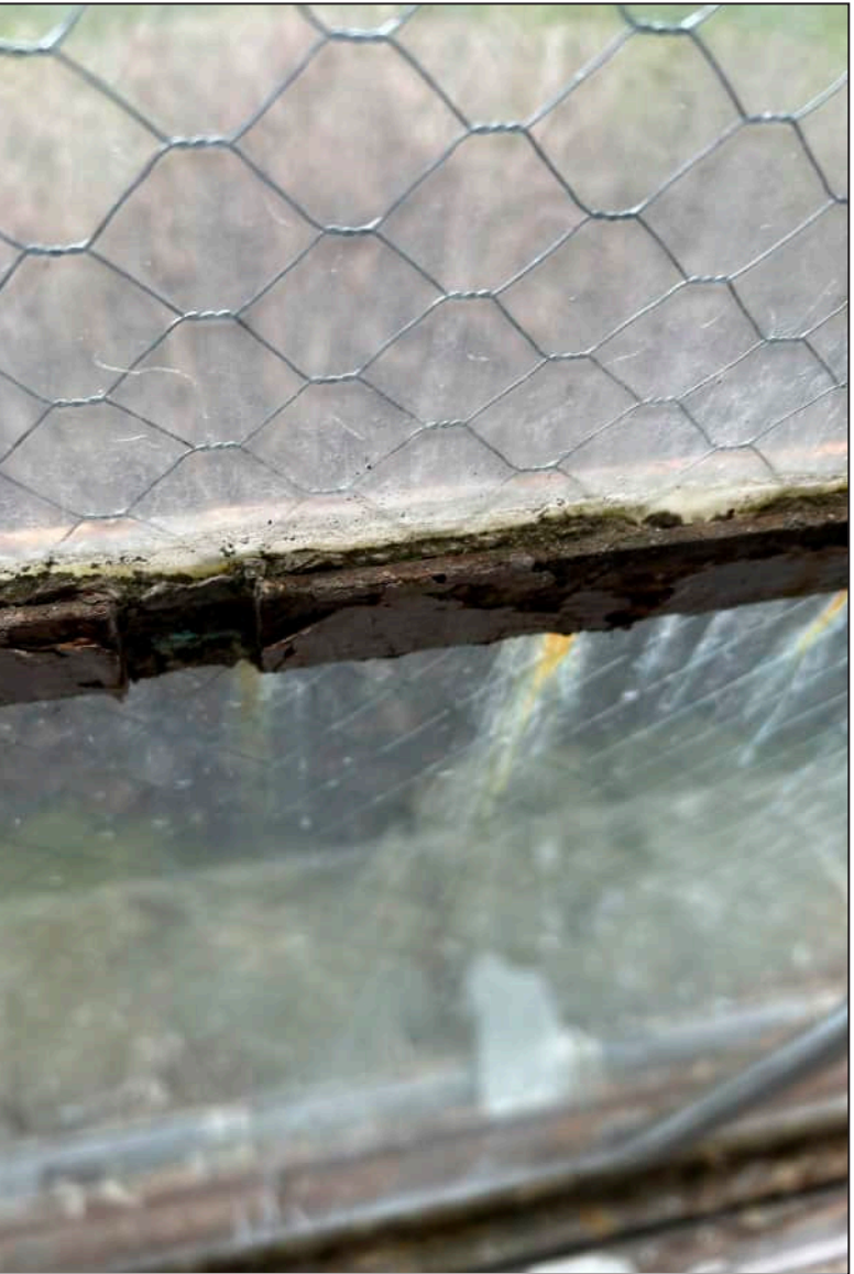
44. W07 – West Elevation, Second Floor, detail of rusting and deterioration at mullion.
