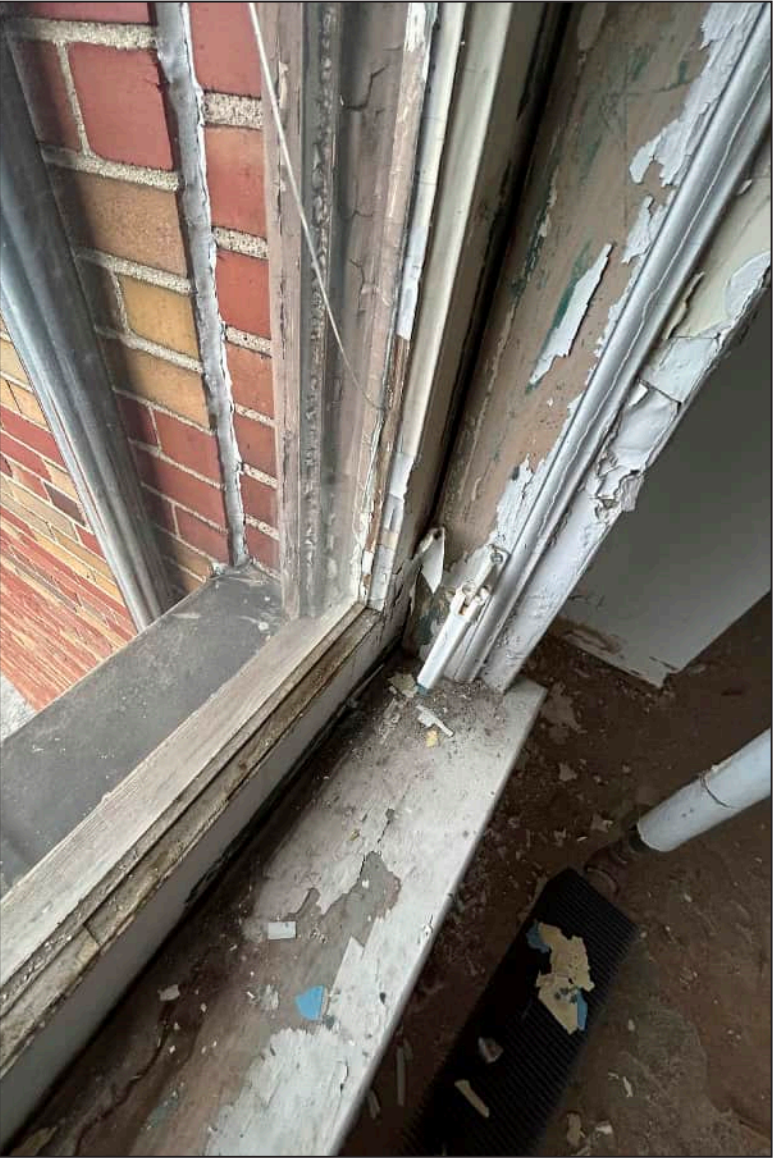
76. N10 – North Elevation, Fifth Floor, detail of deterioration of jamb and bottom sash. Note deterioration of exterior framework.
