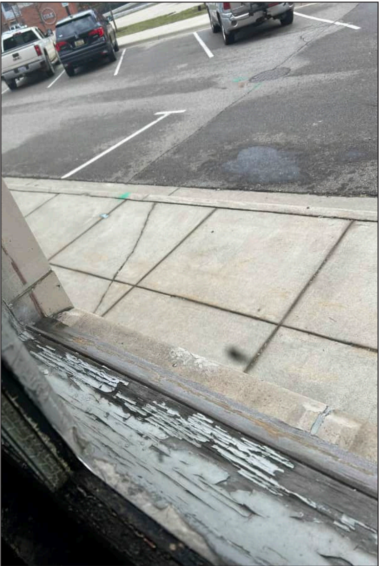
91. E14 – East Elevation, First Floor, detail of exterior sill deterioration.
