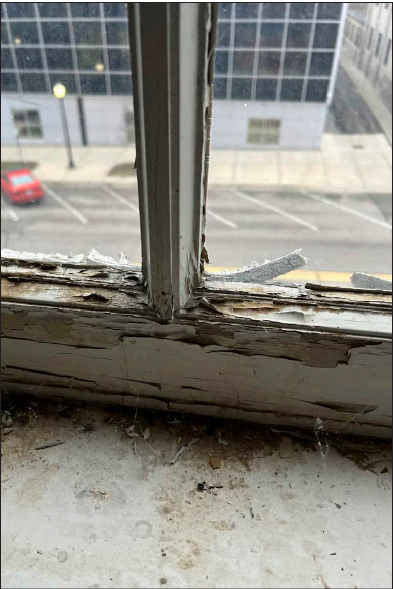
21. S21 – South Elevation, Fourth Floor, detail of rotting at bottom sash. Note separation between mullion and bottom sash.
