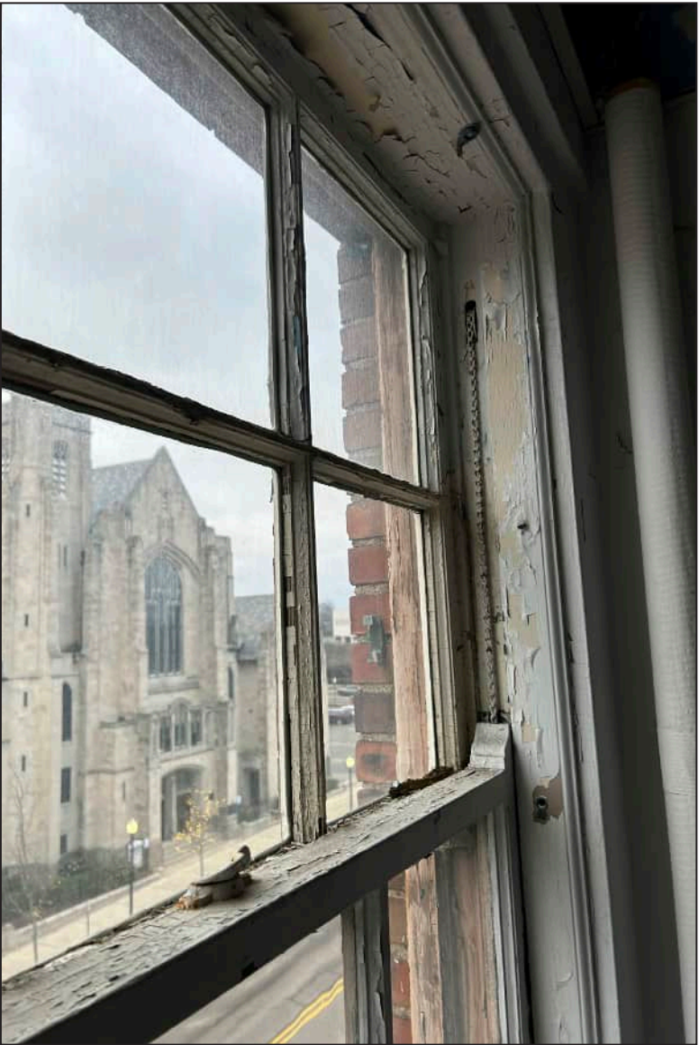
24. S24 – South Elevation, Fifth Floor, detail view of rotting throughout mullions, meeting rail, jamb, and upper sash.
