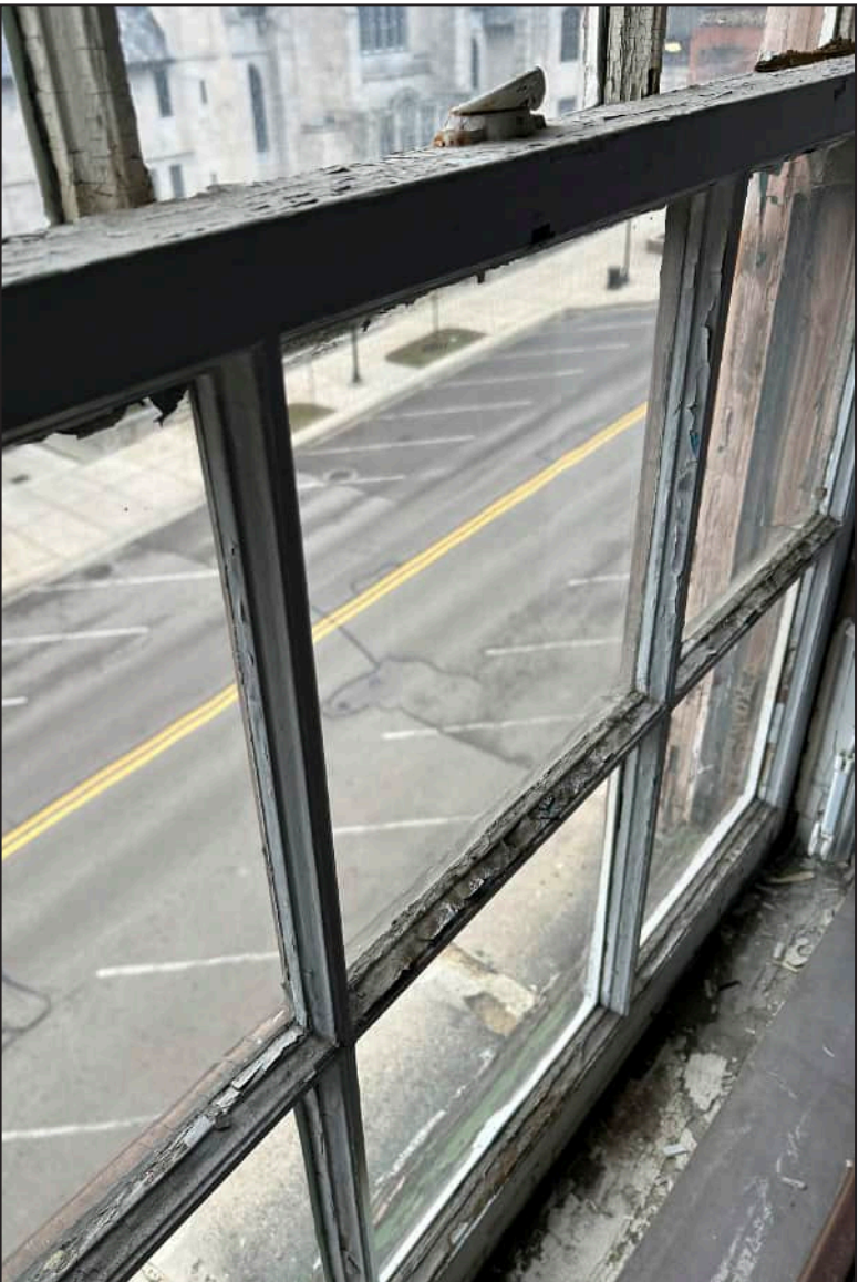
25. S25 – South Elevation, Fifth Floor, detail of deterioration of mullions and general rotting throughout.
