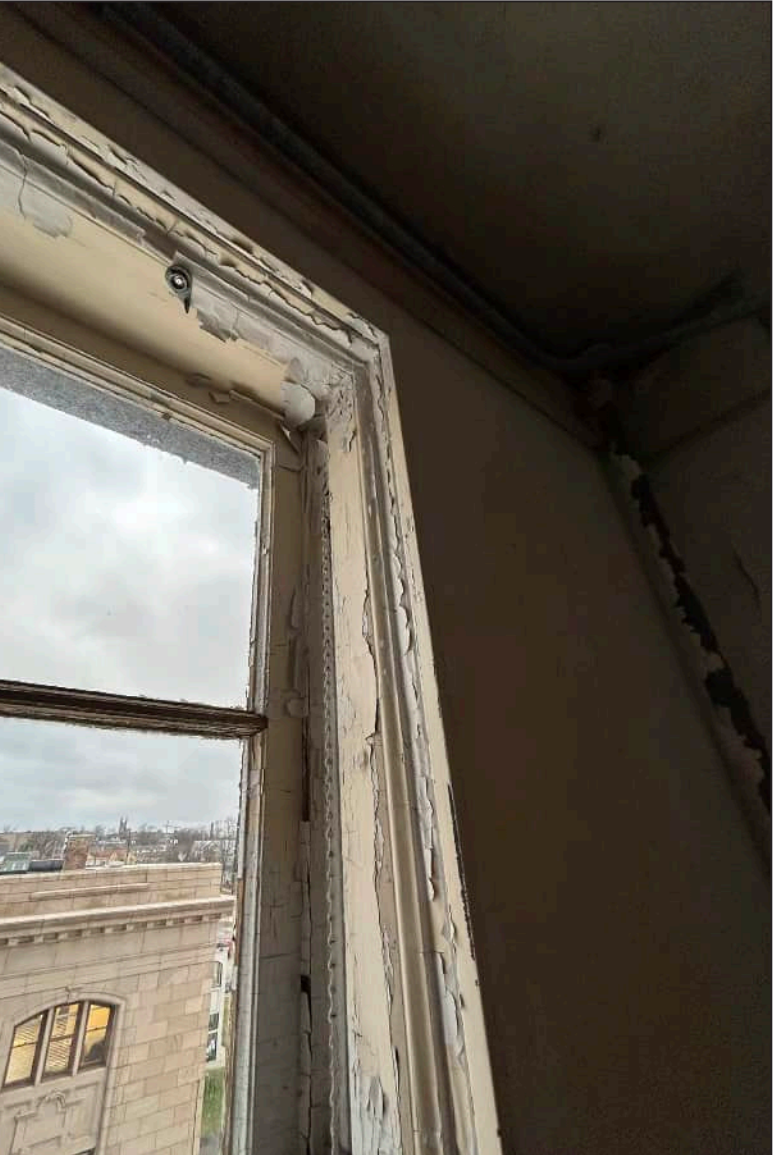
58. W21 – West Elevation, Fifth Floor, detail of deterioration at jamb, upper sash, and mullion.
