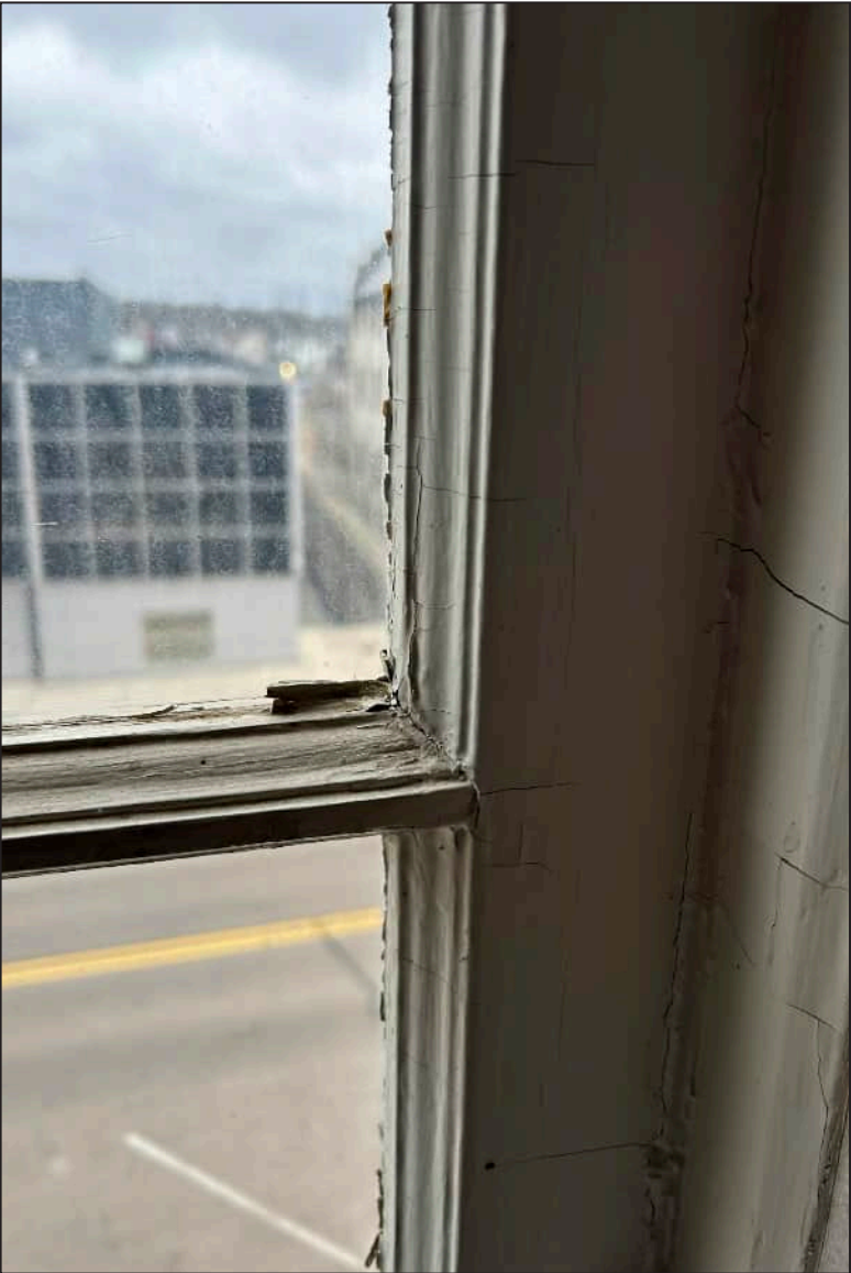
15. S15 – South Elevation, Fourth Floor, detail view of deteriorated mullions, general rotting throughout the framework.
