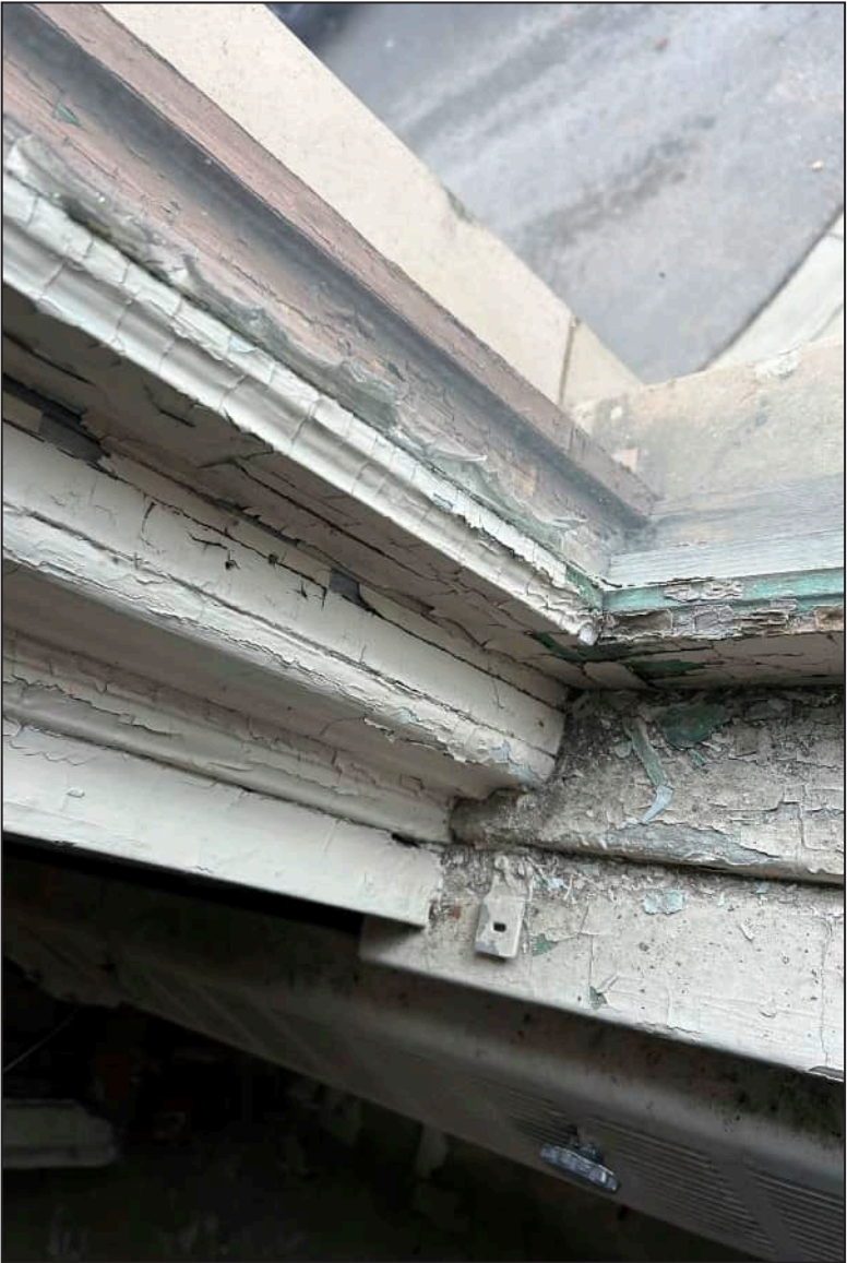
87. E10 – East Elevation, First Floor, detail of deterioration of jamb and bottom sash. Note deterioration of exterior framework.
