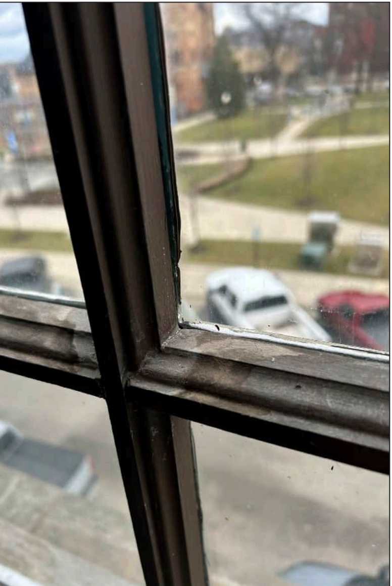
92. E15 – East Elevation, Third Floor, detail of deterioration at mullions.
