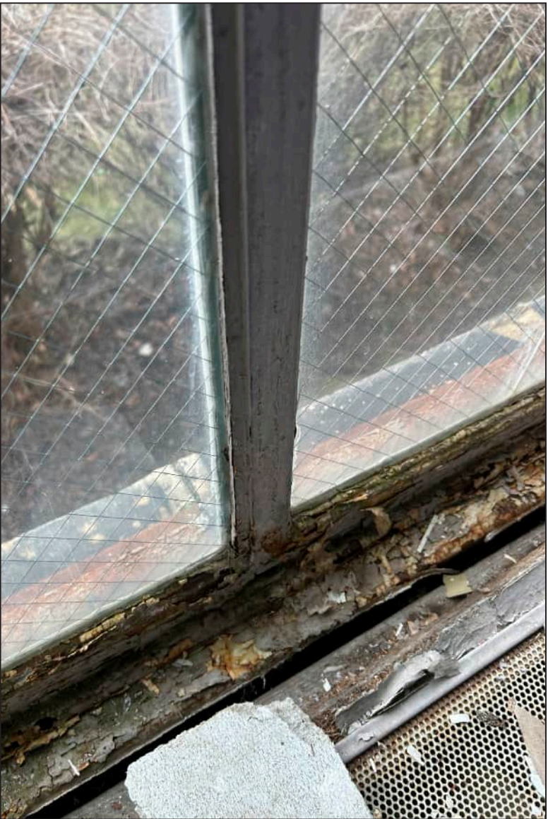
41. W04 – West Elevation, Second Floor, detail of deterioration at bottom sash. Note separation of bottom sash with sill.
