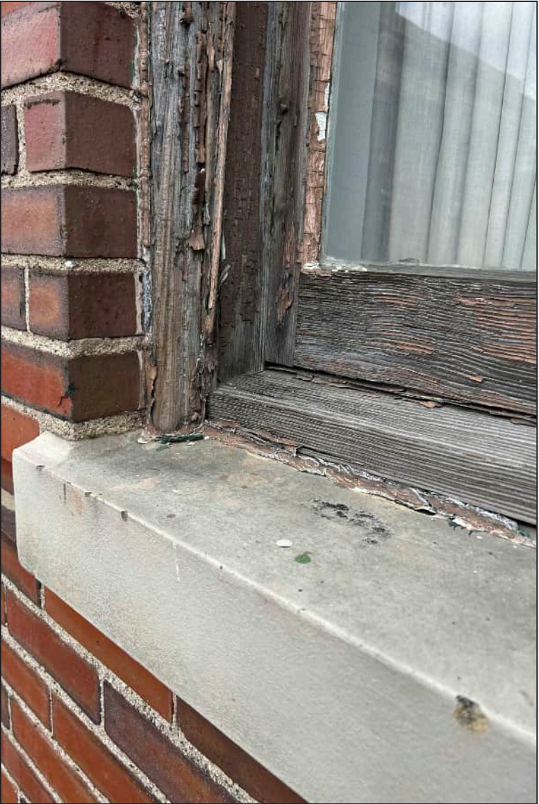
50. W13 – West Elevation, Second Floor, detail of deterioration and rotting at exterior framework.
