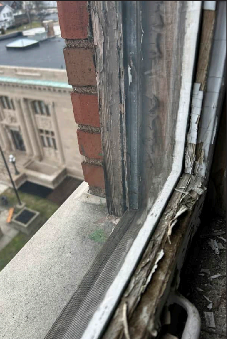
64. W27 – West Elevation, Eighth Floor, detail of deterioration of jamb and bottom sash. Note deterioration of exterior framework.
