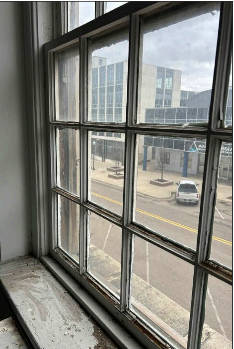
4. S04 – South Elevation, Third Floor, detail view of deteriorated mullions, general rotting throughout the framework.
