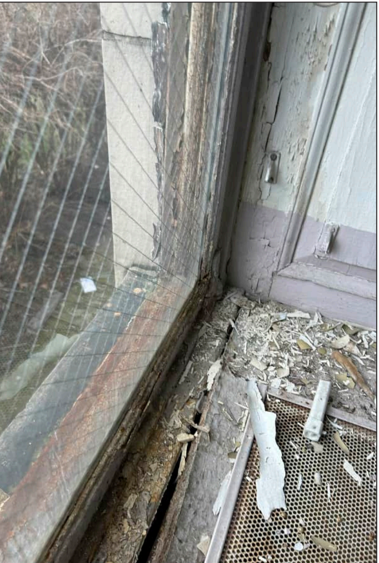
40. W03 – West Elevation, Second Floor, detail of deterioration at jamb and bottom sash. Note separation of bottom sash with sill.
