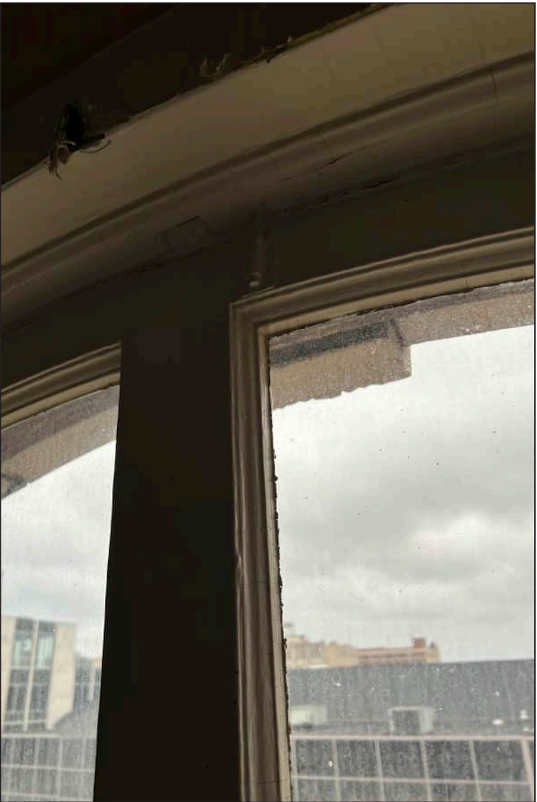
13. S13 – South Elevation, Fourth Floor, detail of cracked casing.
