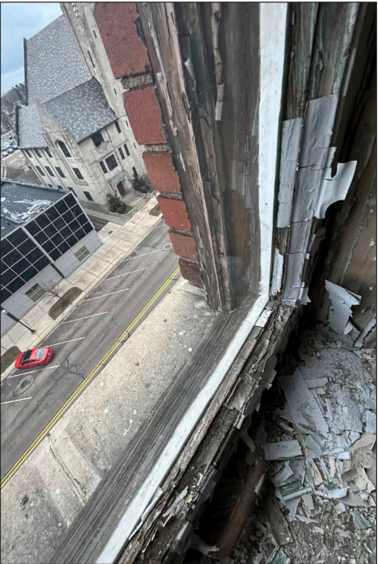
33. S33 – South Elevation, Sixth Floor, detail of deterioration of bottom sash and jamb. Note deterioration at exterior framework.
