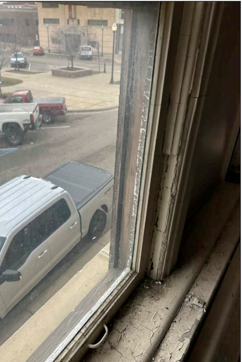
80. E03 – East Elevation, First Floor, detail of deterioration of jamb and bottom sash. Note deterioration of exterior framework.
