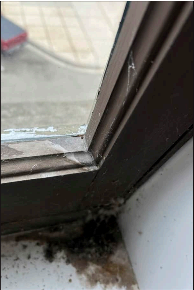
93. E16 – East Elevation, Third Floor, detail of deterioration of jamb and bottom sash.
