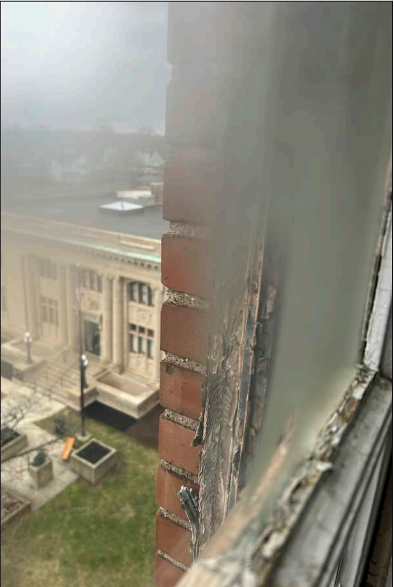
65. W28 – West Elevation, Eighth Floor, detail of deterioration of jamb and bottom sash. Note deterioration of exterior framework.
