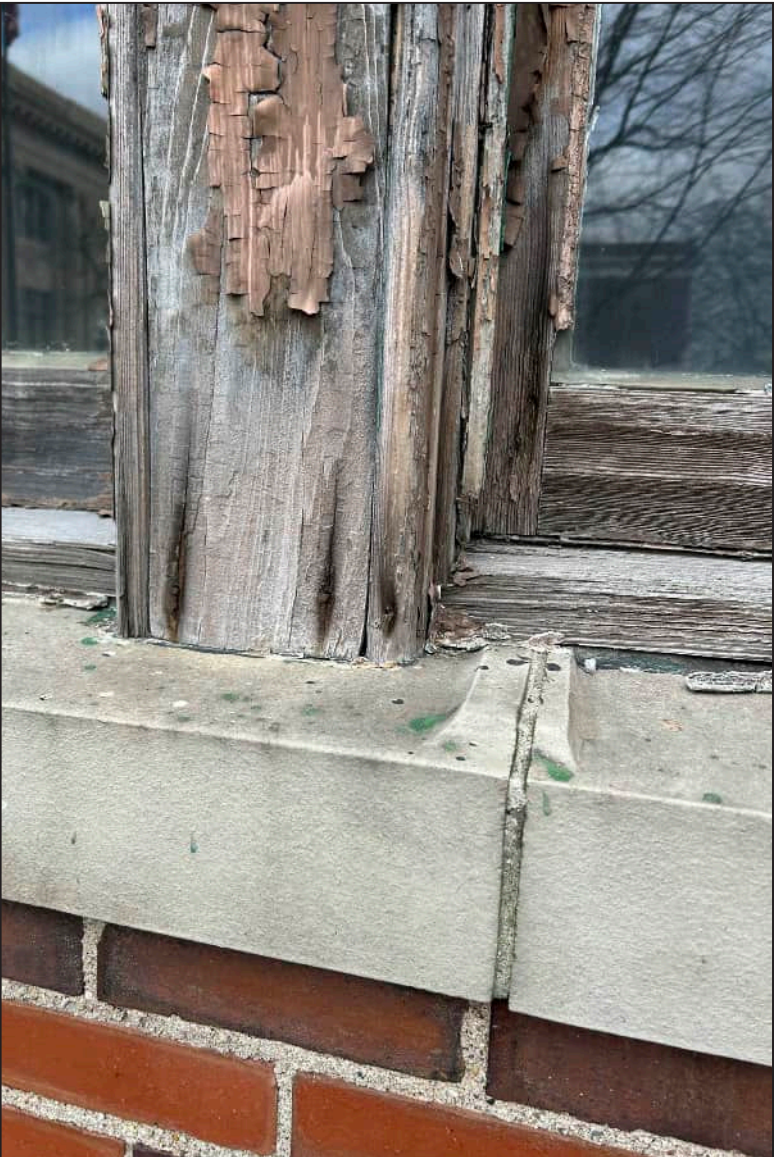
53. W16 – West Elevation, Second Floor, detail of deterioration and rotting at exterior framework and center muntin.
