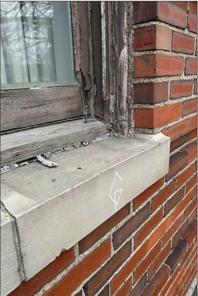
51. W14 – West Elevation, Second Floor, detail of deterioration and rotting at exterior framework.
