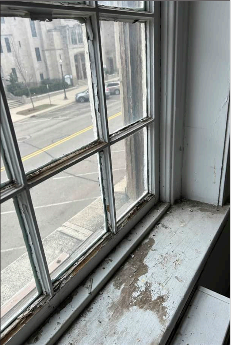
5. S05 – South Elevation, Third Floor, detail view of deteriorated mullions, general rotting throughout the framework.
