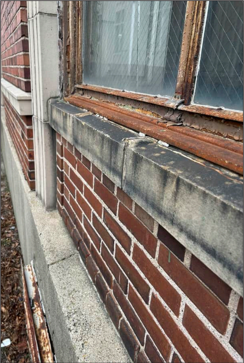
48. W11 – West Elevation, Second Floor, detail of rusting at exterior mullions and framework.
