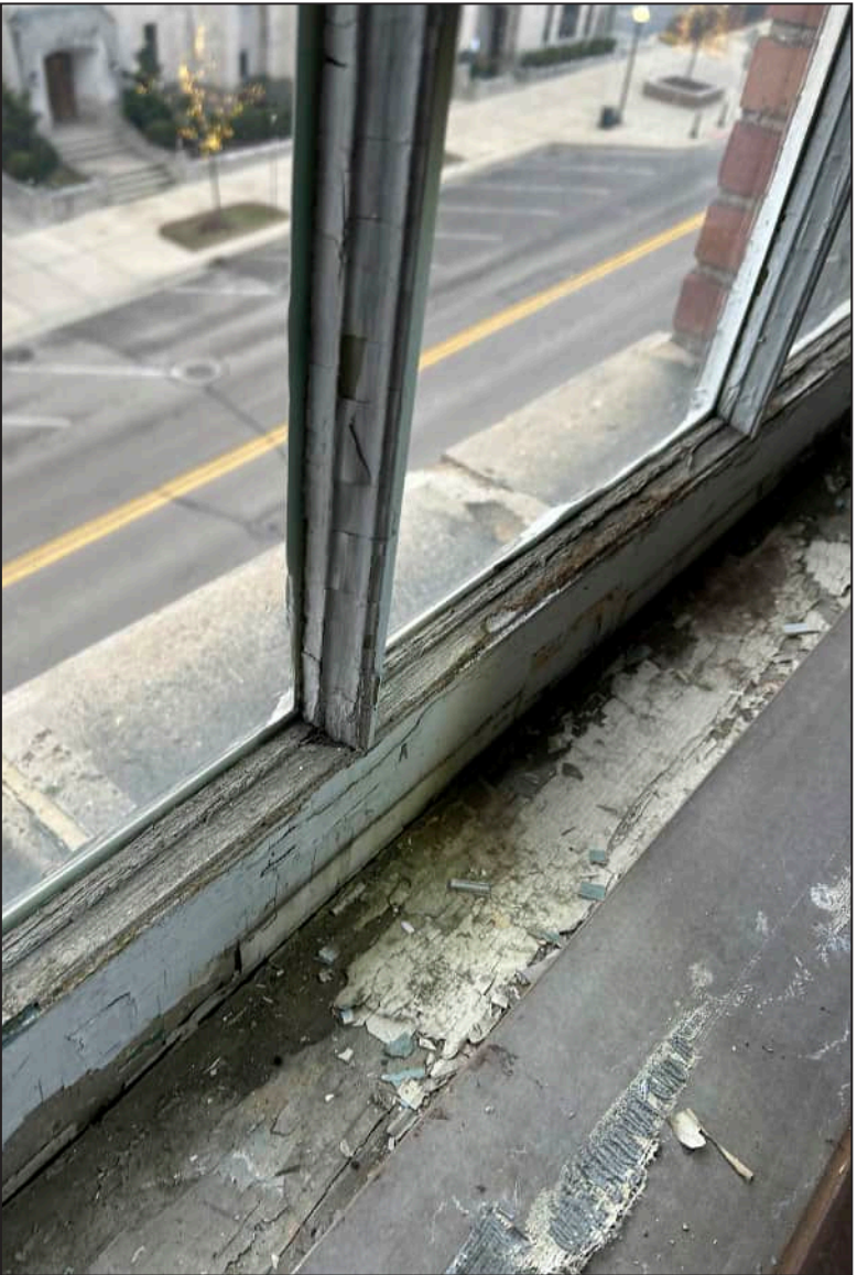
26. S26 – South Elevation, Fifth Floor, detail of deterioration of mullions, separation of mullions and bottom sash, rotting throughout bottom sash, and warped due to weathering and water infiltration.
