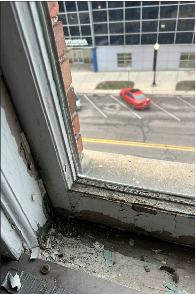
23. S23 – South Elevation, Fifth Floor, detail of rotting at bottom sash. Note separation between jamb and bottom sash.
