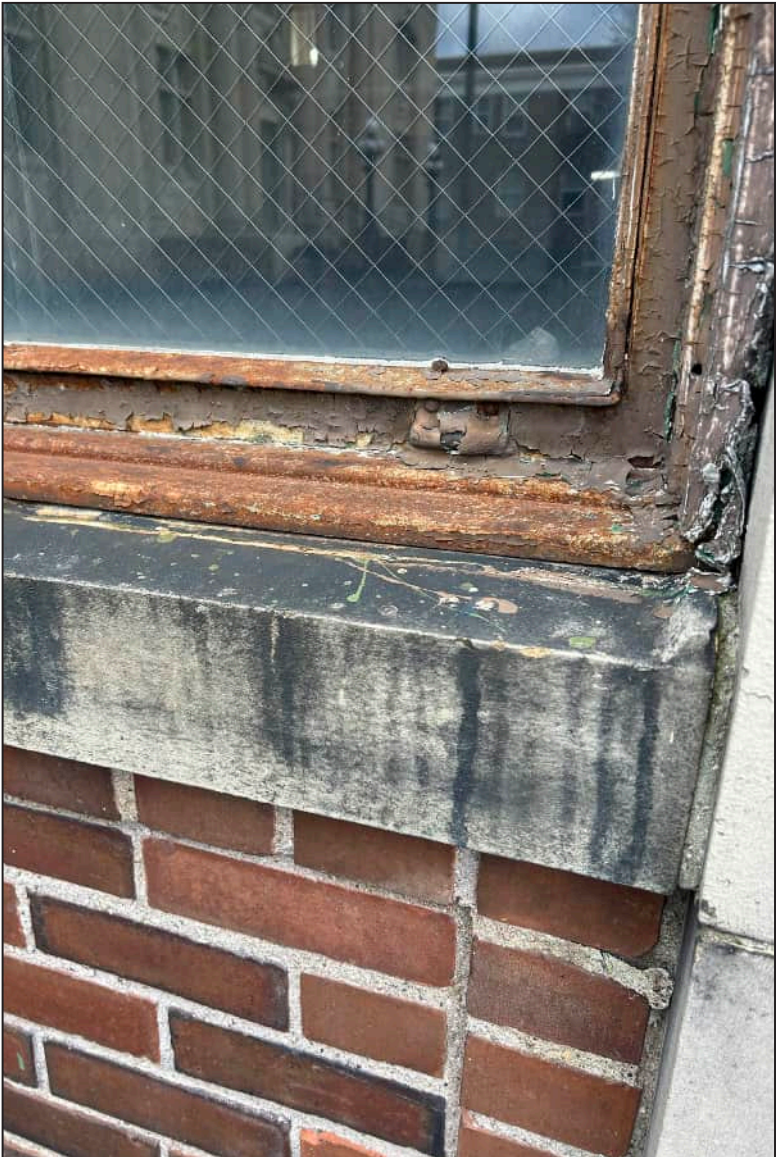
49. W12 – West Elevation, Second Floor, detail of rusting at exterior framework.
