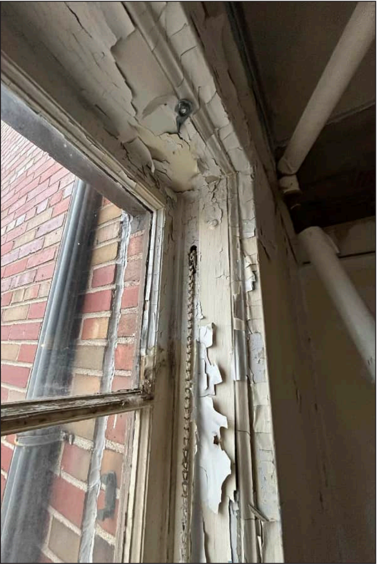
75. N09 – North Elevation, Fifth Floor, detail of deterioration of mullions, jamb, and upper sash.
