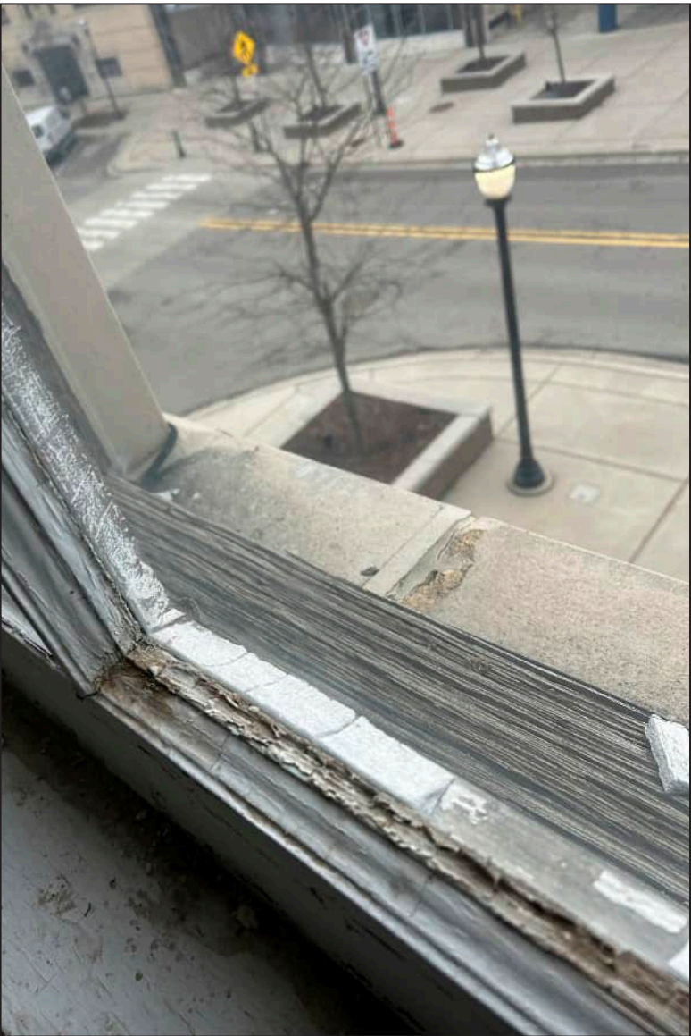
11. S11 – South Elevation, Third Floor, detail of rotting at bottom sash. Note deterioration of wood at exterior framework.
