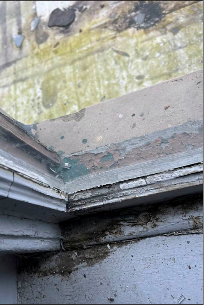
74. N08 – North Elevation, Fifth Floor, detail of deterioration of jamb and bottom sash. Note deterioration of exterior framework.
