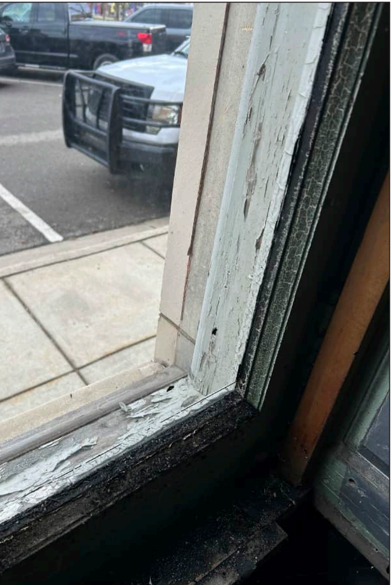
90. E13 – East Elevation, First Floor, detail of deterioration of jamb and bottom sash.
