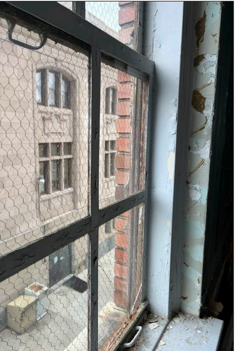
68. N02 – North Elevation, Third Floor, detail of deterioration of mullions, jamb, and bottom sash.
