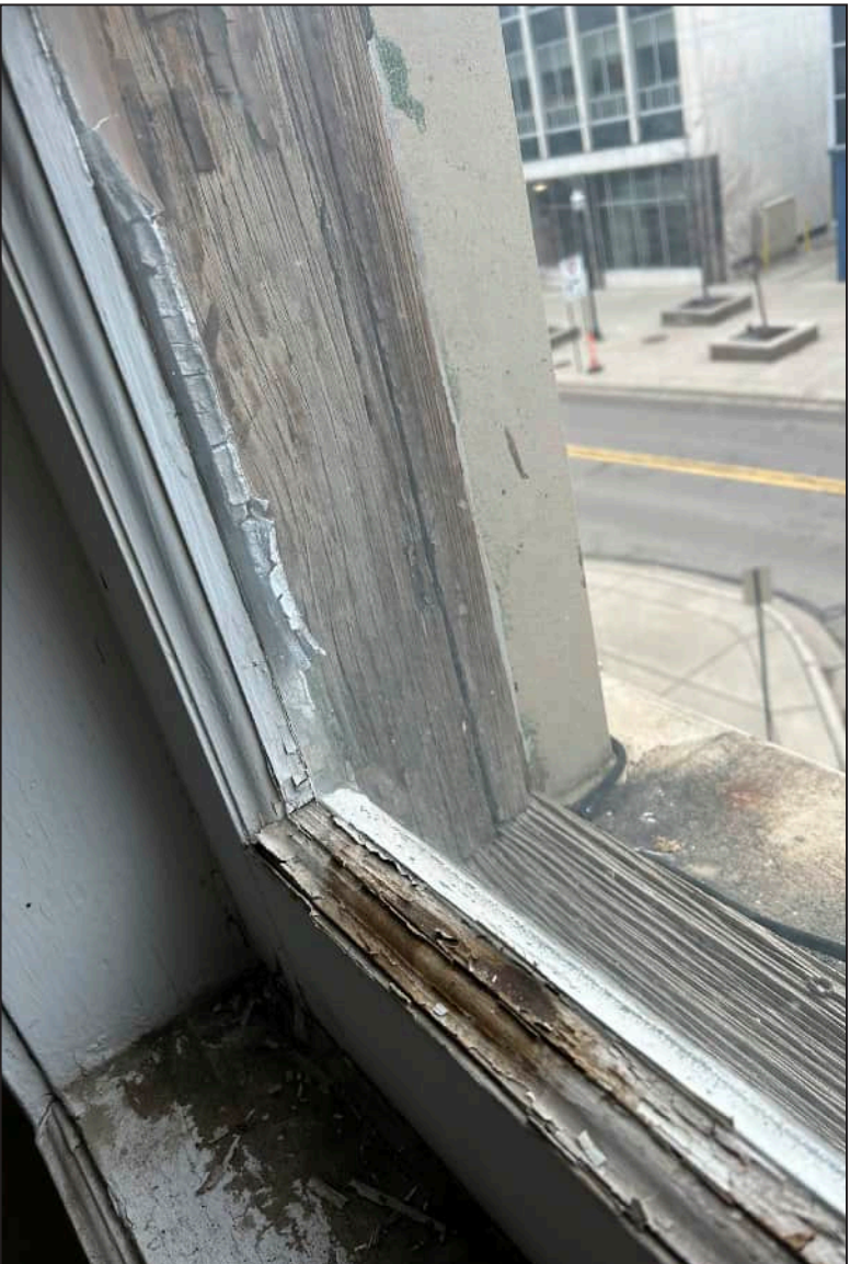
7. S07 – South Elevation, Third Floor, detail of rotting at bottom sash. Note deterioration of wood at exterior framework.
