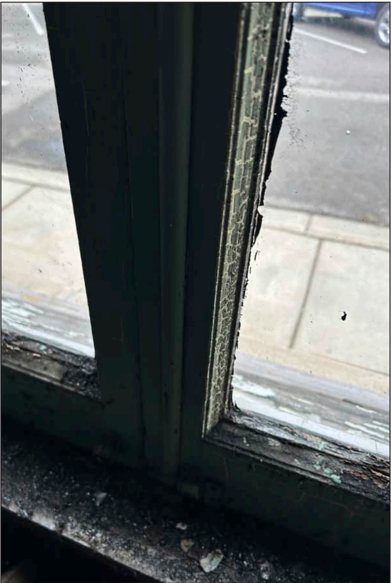
89. E12 – East Elevation, First Floor, detail of deterioration of muntin.
