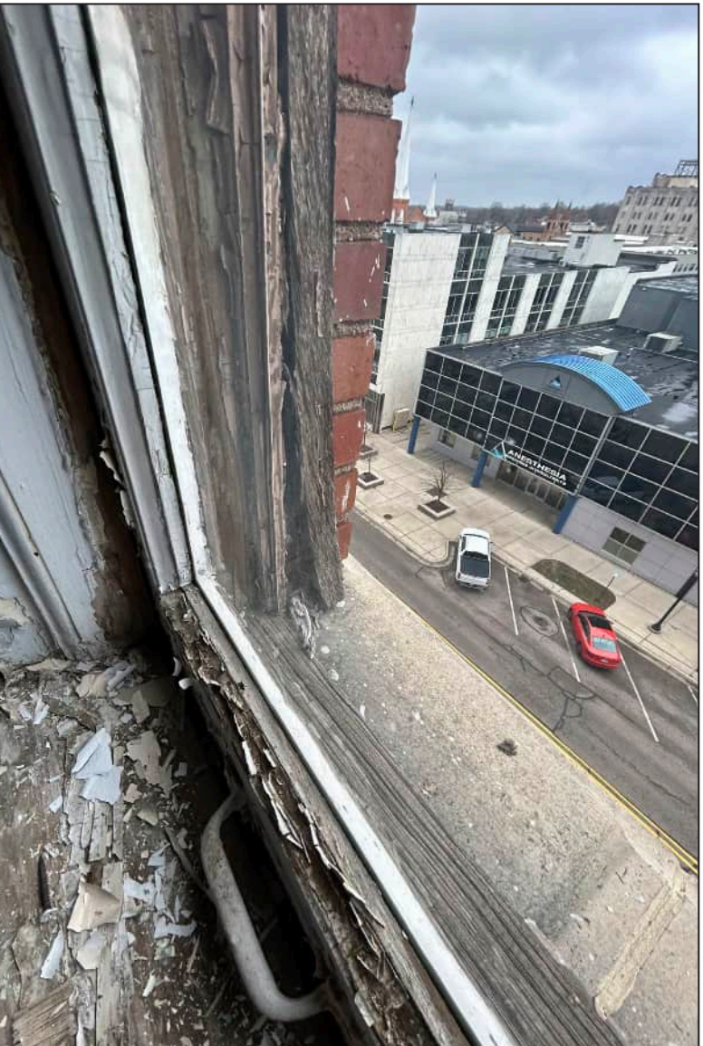
32. S32 – South Elevation, Sixth Floor, detail of deterioration of jamb, bottom sash, and exterior framework.
