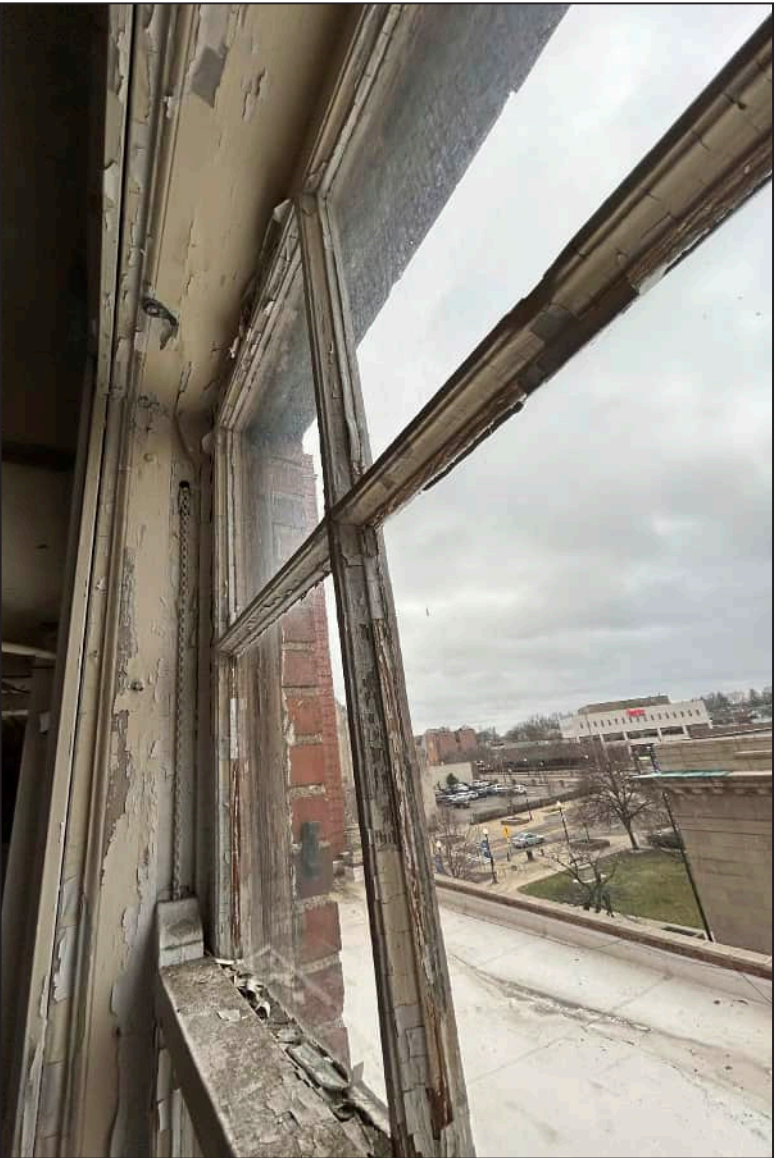
59. W22 – West Elevation, Fifth Floor, detail of deterioration at jamb, upper sash, and mullion.
